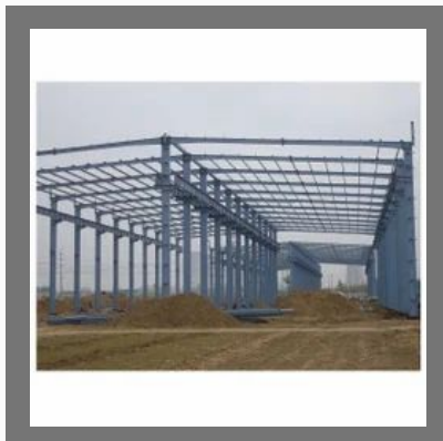
Steel PEB Structural Shed
