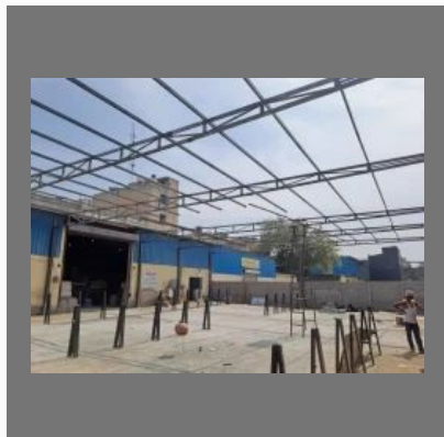
Fabrication Works Teen Shed
